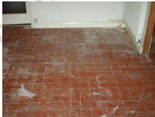
Picture shows Quarry Tile before cleaning and sealing.
